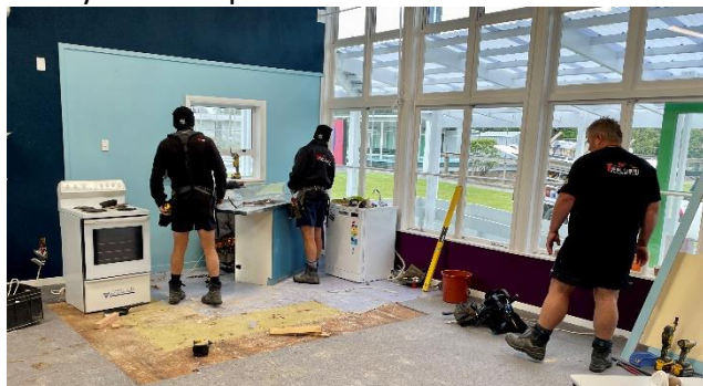
Wayne Stewart Building and Contracting reconfigure the kitchen unit in the staff room
